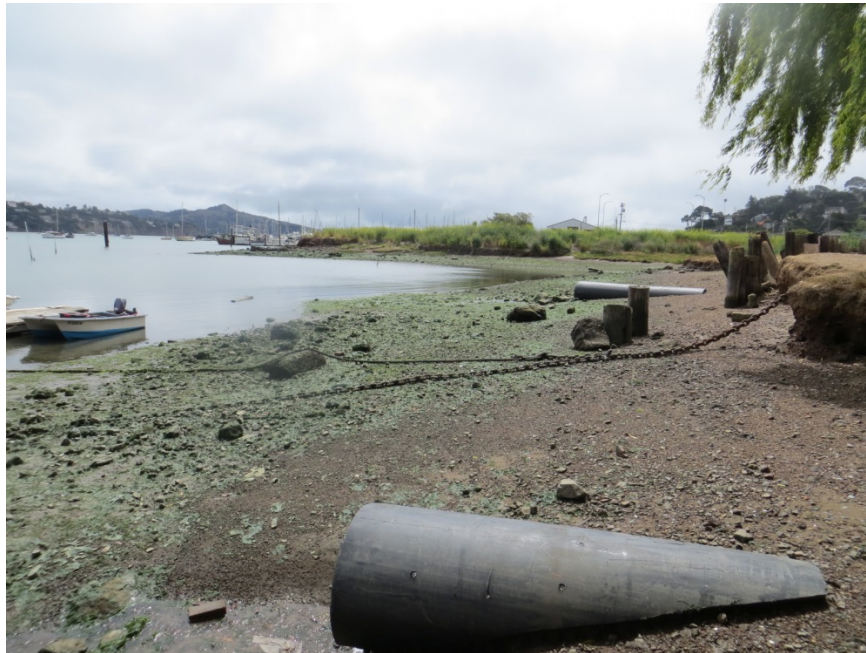
Figure 3. Two stormdrain outfalls currently drain in the tidal access area. These are corroded corrugated pipes that have been temporarily covered with PVC to protect the public. The outfall closer to the public access point will be removed, and the other will be replaced with a more stable long-term solution.
